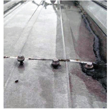
Loose or Missing Fasteners
